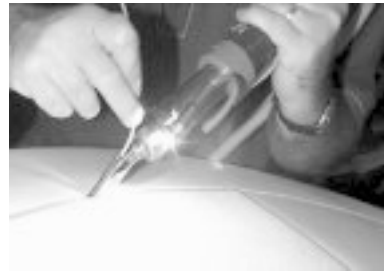
Figure 8.26 Hot-gas welding of fabric-backed fluoropolymer sheets prior to laminating. (Courtesy CPF Dualam.)
