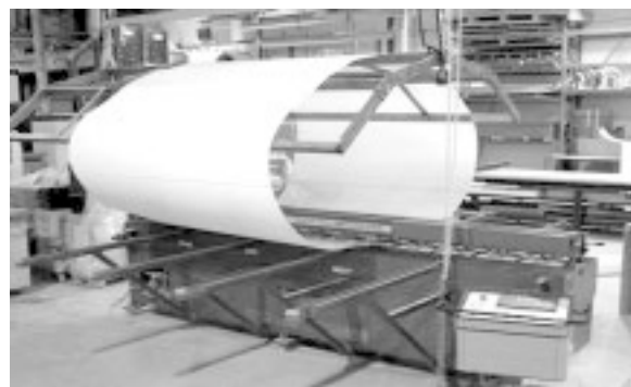
Figure 8.22 Machine butt welding of fluoropolymer prior to dual laminate construction. (Courtesy CPF Dualam, Montreal, Canada.)
