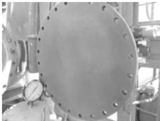
Figure 4.2. Photograph of a typical lined manway. (Courtesy DuPont Engineering Technology.)
