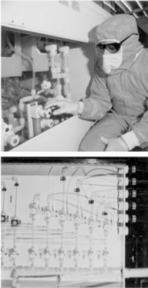
Figure 6.23 Extruded PFA tubes in a high purity fluid handling system. (Courtesy Advanced Micro Devices and DuPont Companies.)
