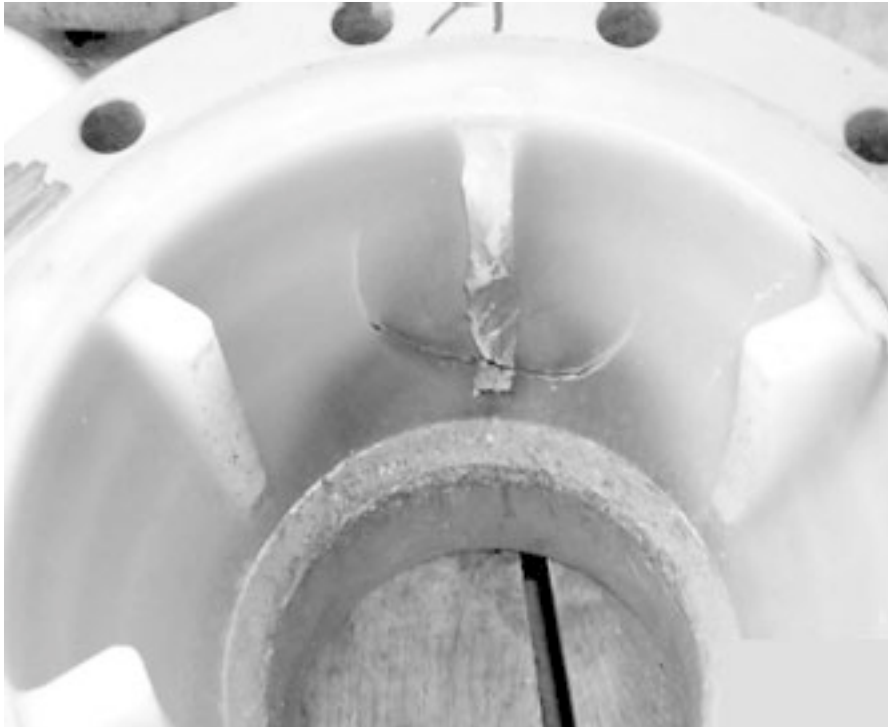
Figure 10.37 Photograph of the PFA-lined valve body (Case 2). (Courtesy DuPont Company.)
